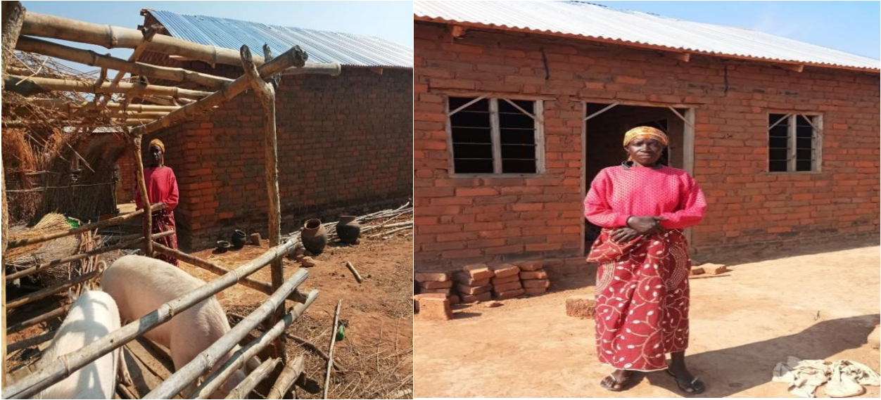
Plate 7: A house built by a beneficiary after selling pigs in Mawande, Makambako
